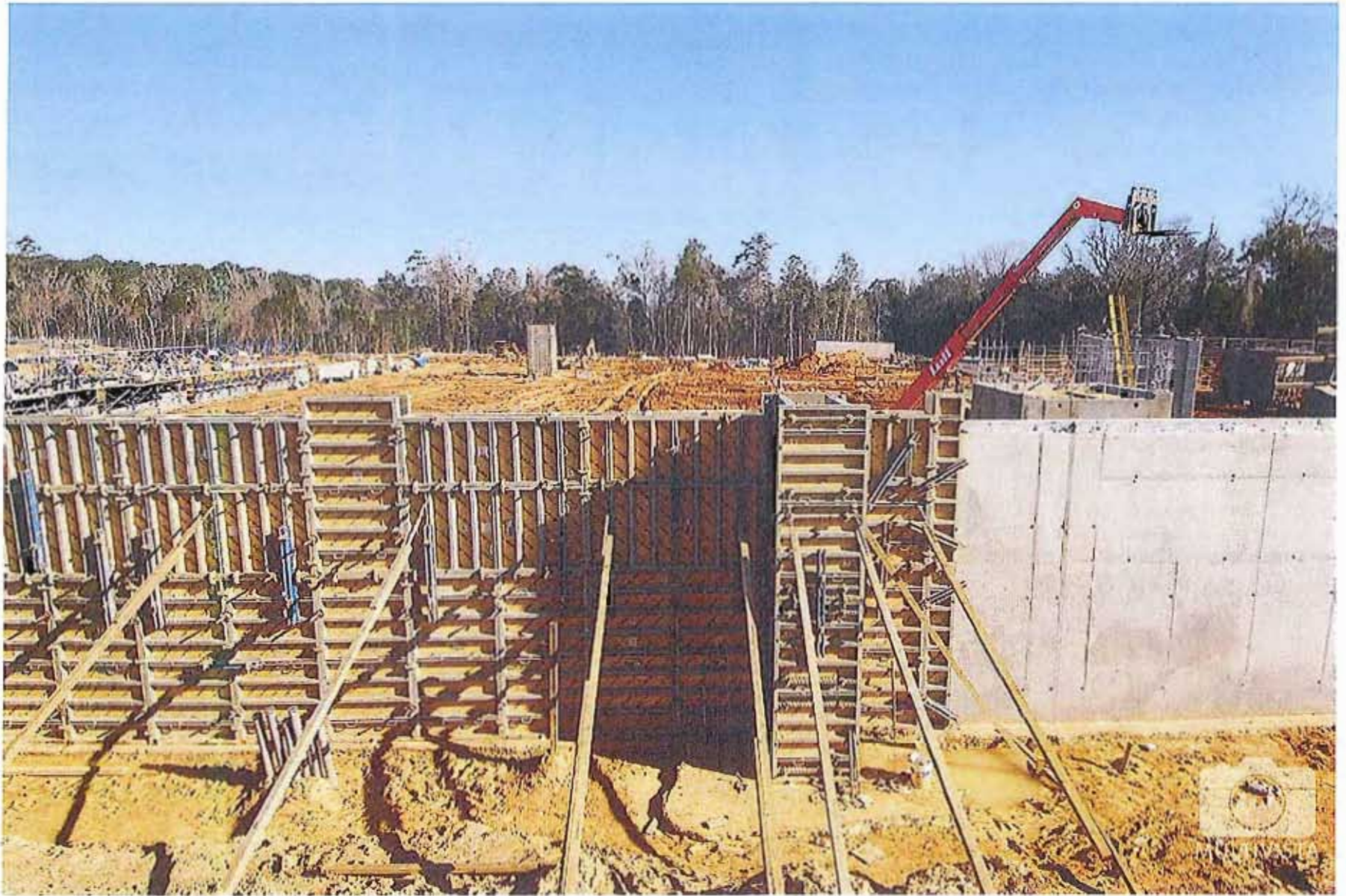
Tallahassee Community College - TCC Ghazvini Center for Healthcare Education - 1628 Surgeons Dr - Exterior Progression - - February 17 2010 - Photo Number 6
